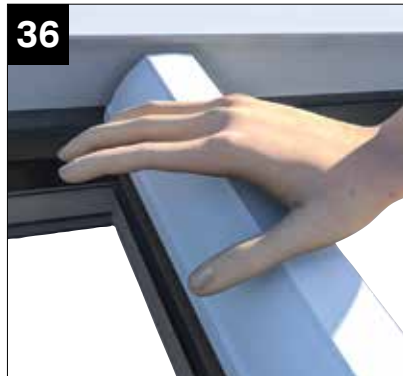
36 Using the heel of your hand, push down on the top cap to engage the clips, working from ridge to rider rail. Ensure the rubber gaskets are fully compressed for a watertight seal. NOTE: on longer bars it may be necessary to use a soft mallet and timber block.
